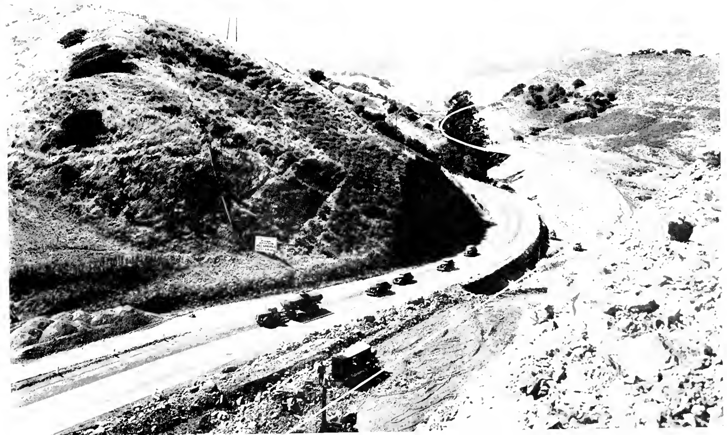
Scenes on realignment construction of U. S. 101 south of San Luis Obispo. Top picture shows bridge being built and rough grading near San Luis Obispo Creek. Below—White line indicates new route compared with existing grade
